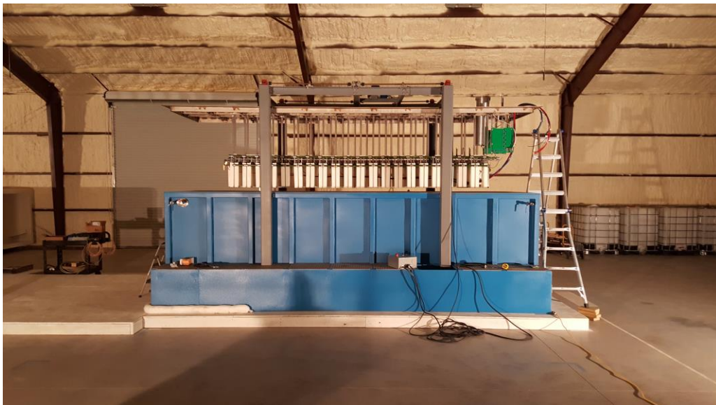
Figure 1. The APELC 4 MV Marx generator.
