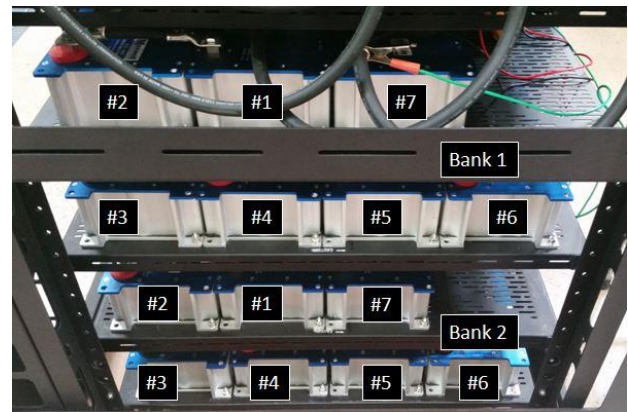
Fig. 5. Configuration of the Ultracapacitors which are serially connected to form each bank.
